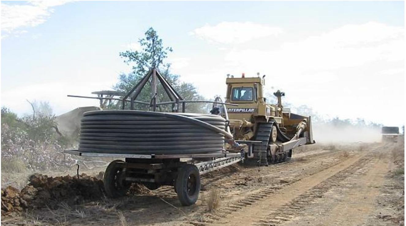
The 3000km of irrigation pipe being laid at Beetaloo station. Source: Supplied
